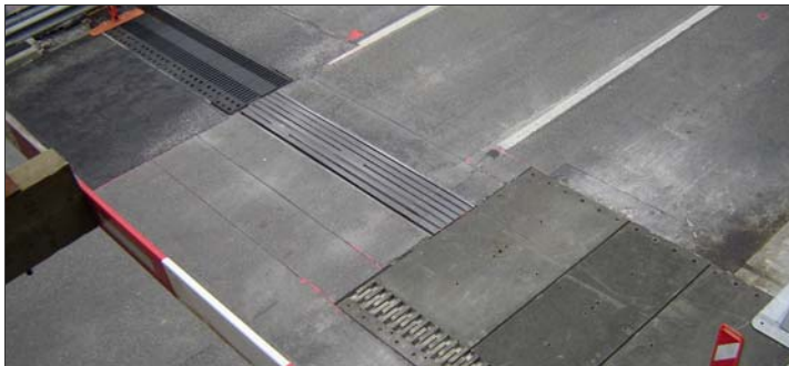
Figure 4: Replacement of existing expansion joint with Tensa®Flex Sliding Finger, using the “Mini-Fly-Over” system to minimise impact on traffic.
