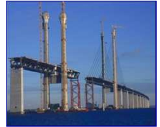
Øresund Bridge (Denmark-Sweden) Pot bearings V_{max} = 96'000 kN
