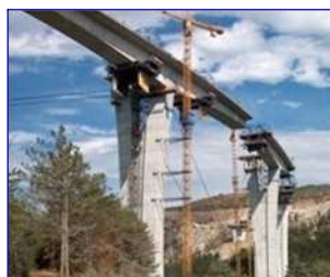
Črni Kal Viaduct (Slovenia) Modular expansion joint type LR9 (720mm)
